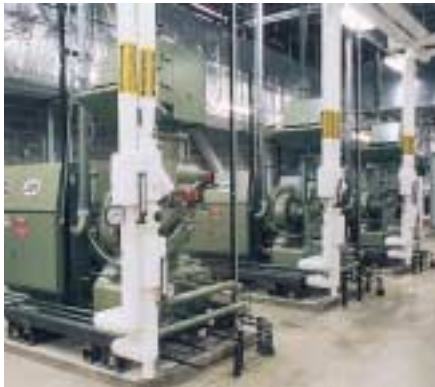
Three 200 HP (150 kW) Turbo Air® Compressors installed at an electronics facility.
