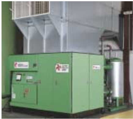
150 HP (112 kW) Air Cooled Turbo Drypak Compressor installed in manufacturing plant. Hot air from air coolers used to heat factory.
